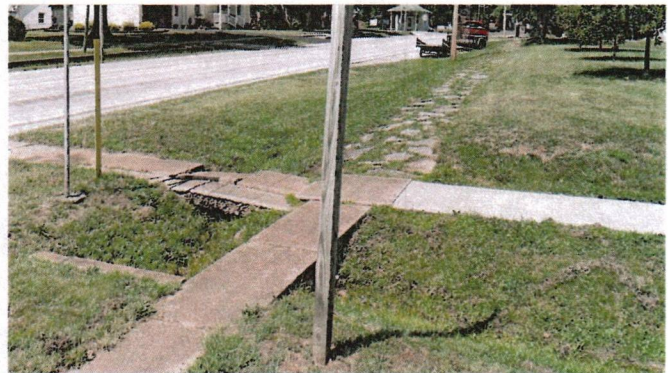
Sidewalk improvements are needed along Butterfield Trail to accommodate all users.
